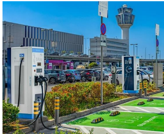
EV charging station
